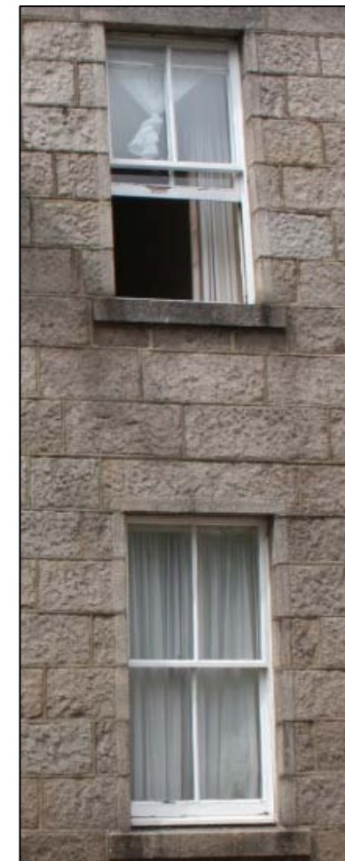
Repair of sash & case windows can often be much cheaper than replacement
